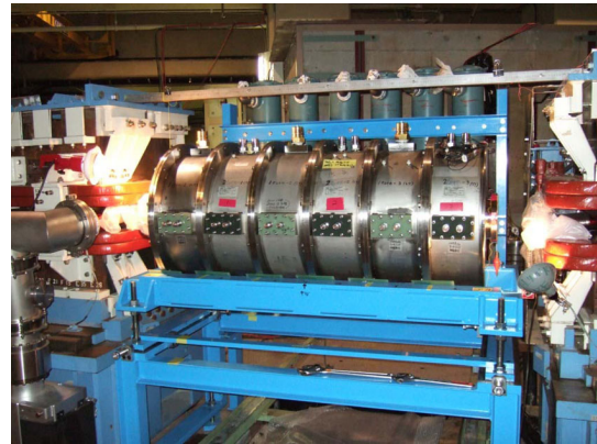
FIG. 30. Acceleration cells installed in the straight section of the KEK-DA.
